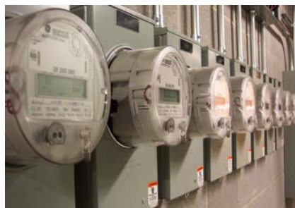
Sub-meters are used to monitor power use by department or floor
